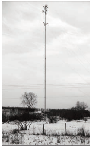
The Sheguiandah tower will be activated by month's end.
