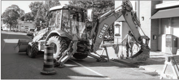
The Northeast Town public works crew repairs a small sinkhole that appeared at the front of the Little Current Post Office late last week.
