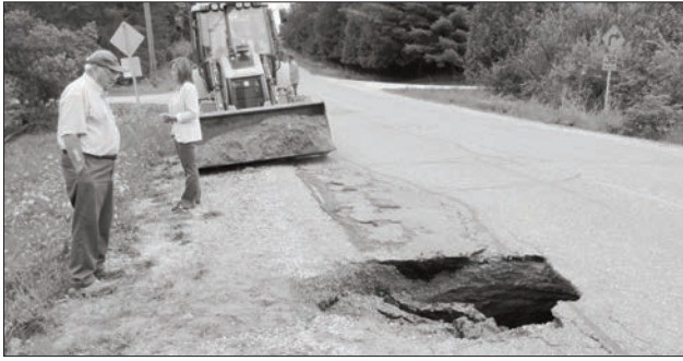
Gore Bay Councillor Harry VanderWeerden and town clerk Annette Clarke view the damage to Highway 540B leading into the town of Gore Bay due to the heavy rainfall Tuesday evening.
