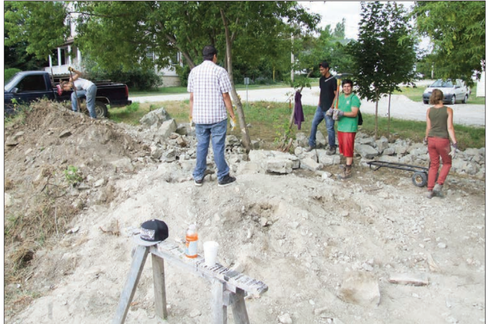
Wwoofers, students, artists and playwrights got into some heavy lifting as they utilized a collection of stones from the renovation of the former Mastin's store in Manitowaning into the Debajehmujig Creation Centre to create an amazing set of raised organic garden beds.
