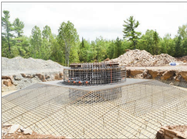
ABOVE: This photo shows the construction of a turbine base from the McLean's Mountain Wind Farm project. After the excavation of the site, a rebar frame is constructed.
