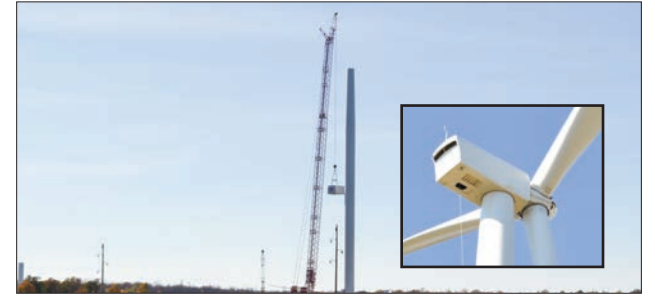
A large crane moves the nacelle to the top of the tower. INSET: The nacelle houses all of the generating components including the generator and gearbox.
