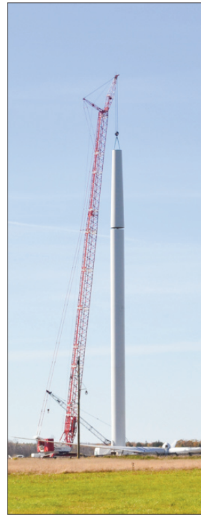
Section five of the tower is slightly tapered at the top, allowing for the nacelle to fit atop.
