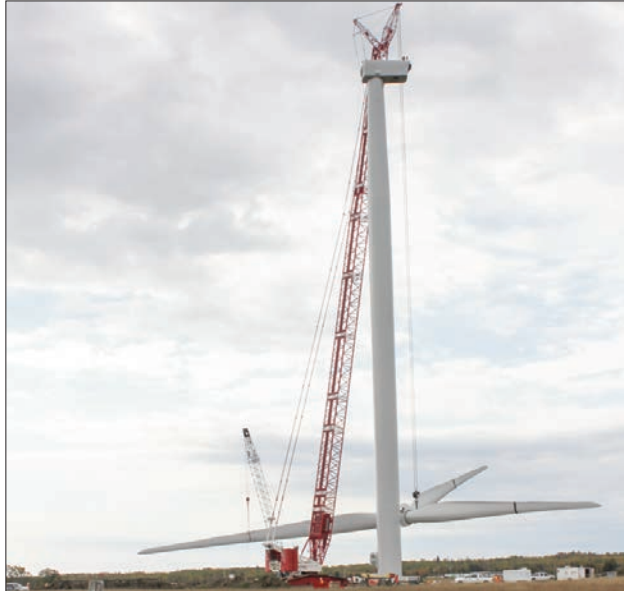
After being assembled on the ground, the rotor is lifted using the two cranes and is attached to the top of the tower.
