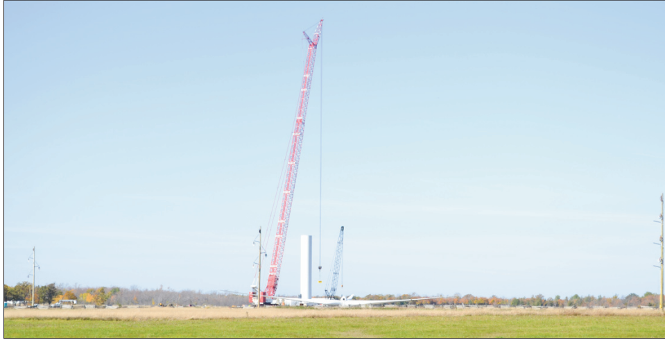
The turbine tower is erected in five sections. The above is to first two sections of the tower T5.
