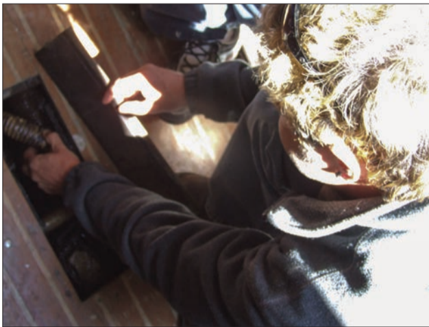
Ray Quenville checks the bilge and hoses of Delirious. No smell of diesel fuel is apparently a very good sign.
