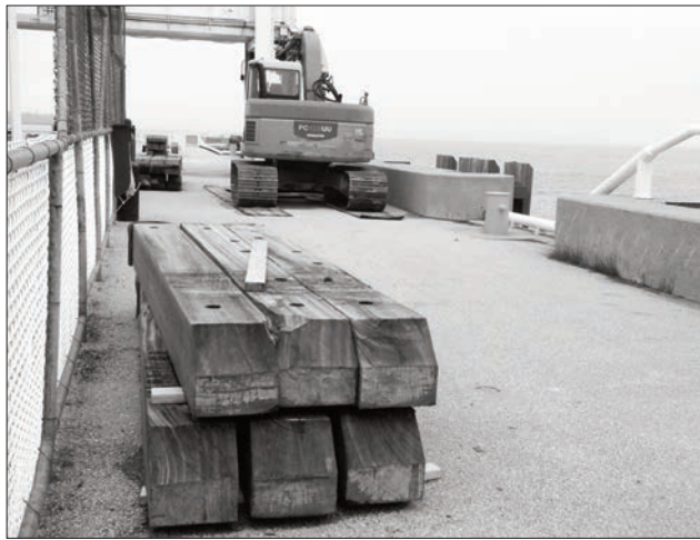
The fender timbers have been removed at both the Tobermory (seen above) and South Baymouth ferry terminals.
