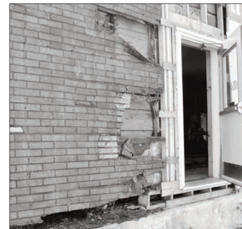
As work proceeded on renovating the Sheguiandah Seniors' Hall it quickly became apparent that there was going to be some very serious work required.
