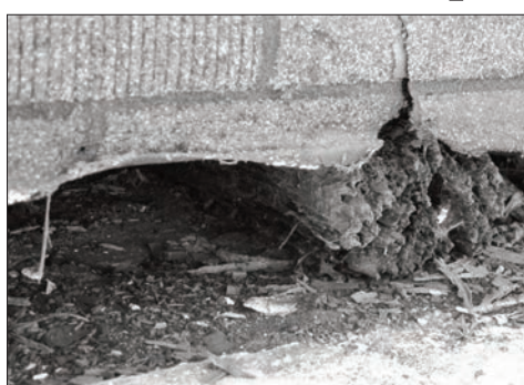
It was originally thought that all the Sheguiandah Seniors' Hall needed was a little tender loving care with some floor joists.
