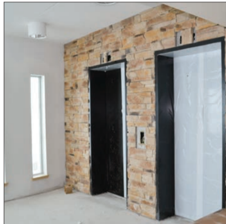
The elevators have been installed and are operational, but are awaiting inspection.
