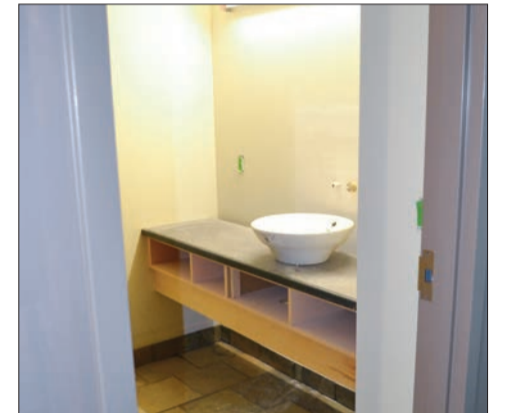
The bathrooms are coming along, with toilets and showers installed on the third and fourth floor and the first and second bathroom's scheduled to have been finished last week.
